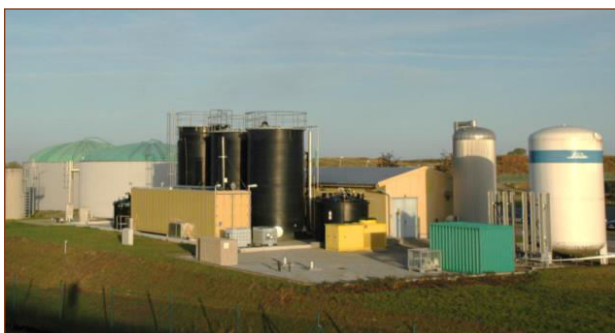
Sickerwasserbehandlungsanlage Leachate treatment plant
