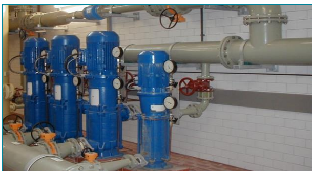
Reinwasserpumpwerk Clean water pump station
