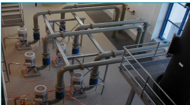
Pumpstation Pumping station
